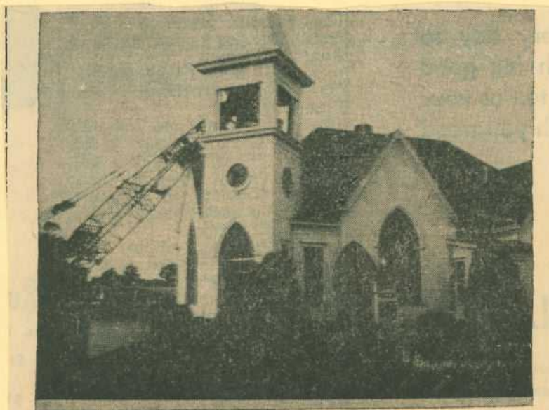
It was a very delicate task but Hall's Contracting of Exeter lifted the bell out of the tower without incident. This bell will again ring, but not until in place in Friend's new Congregational Church
